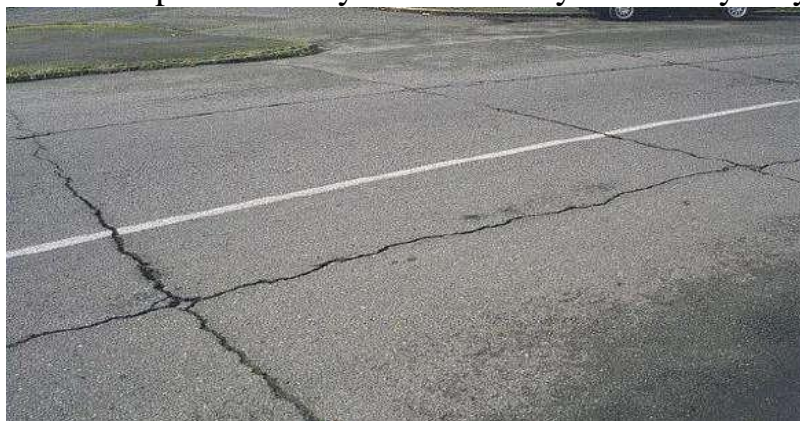
Fig. Joint Reflection Cracks
