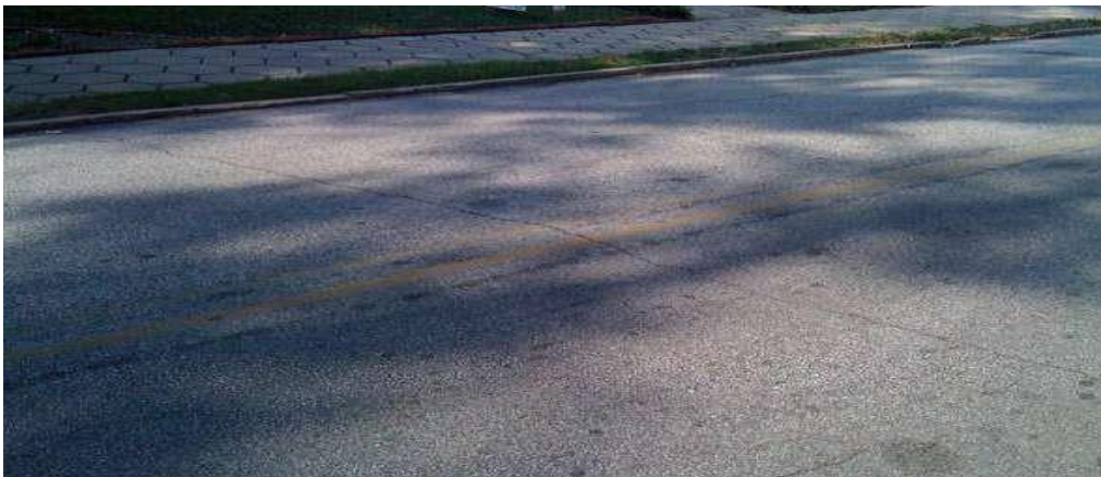
Fig. Transverse Cracking
