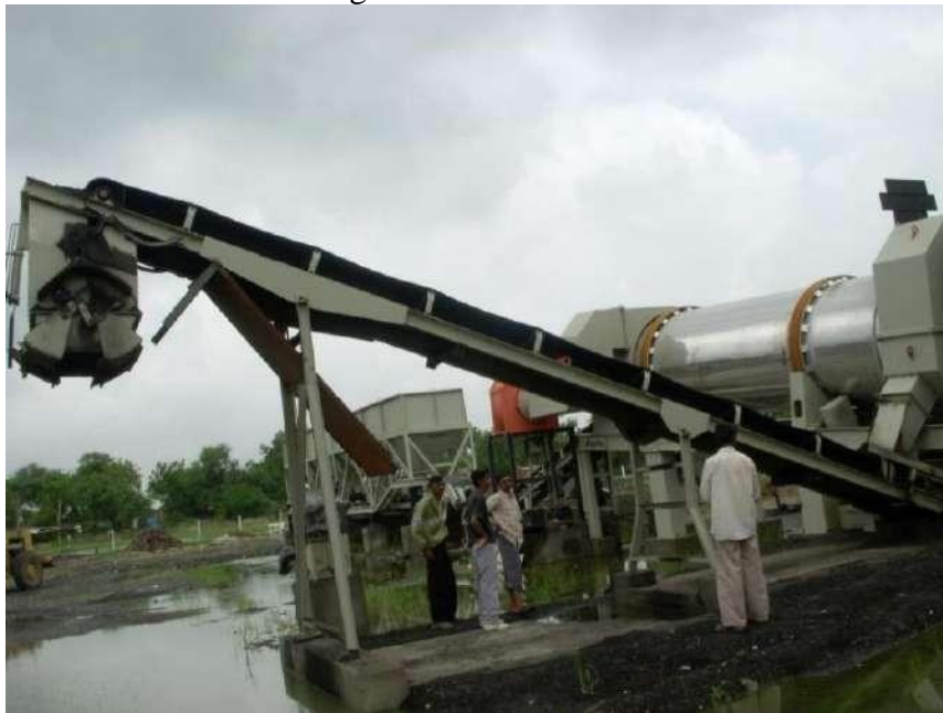
Fig. Load Out Conveyor
