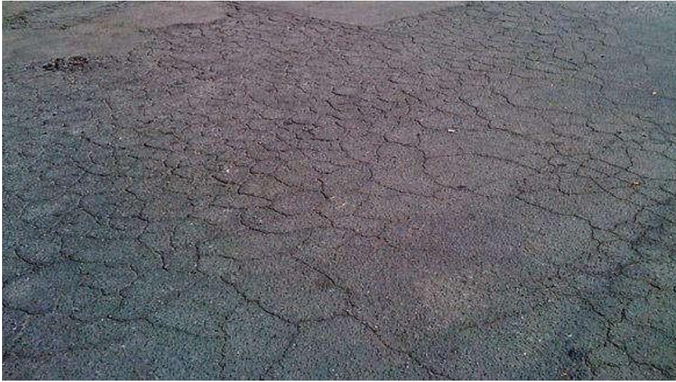
Fig. Alligator Cracking
