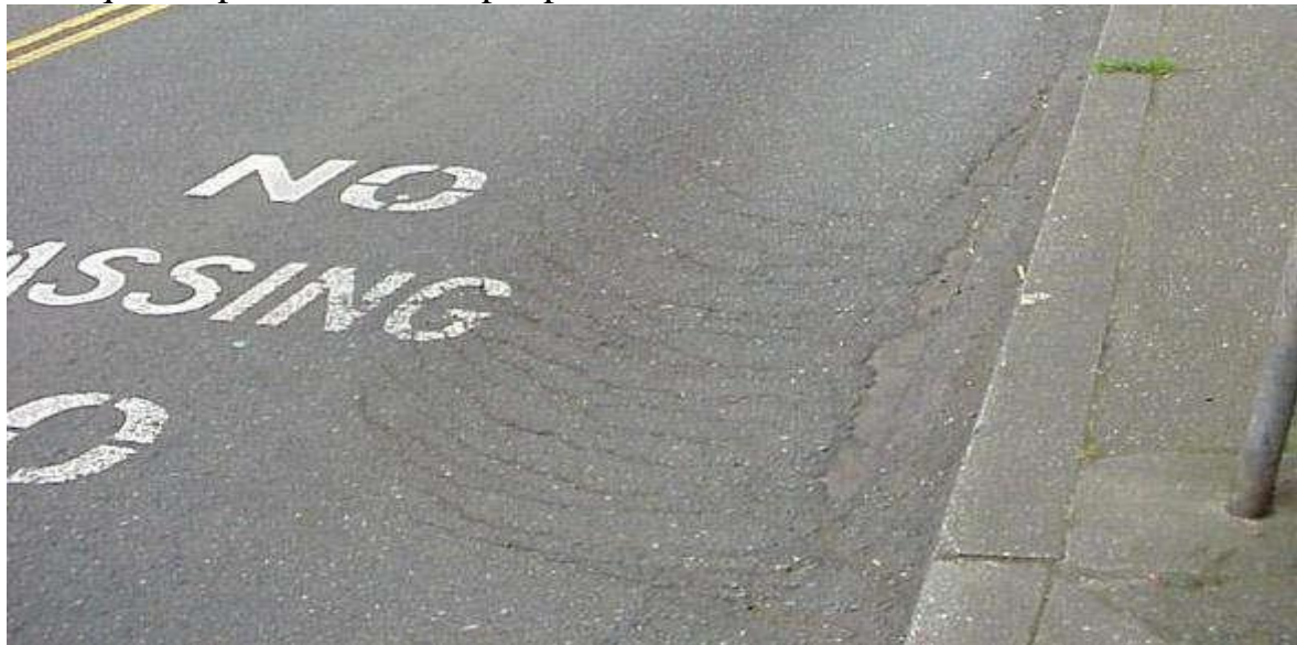
Fig. Slippage Cracks
