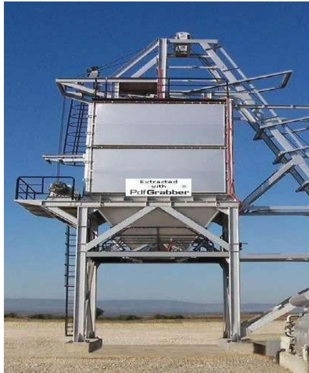
Fig.Hot mix storage silo
