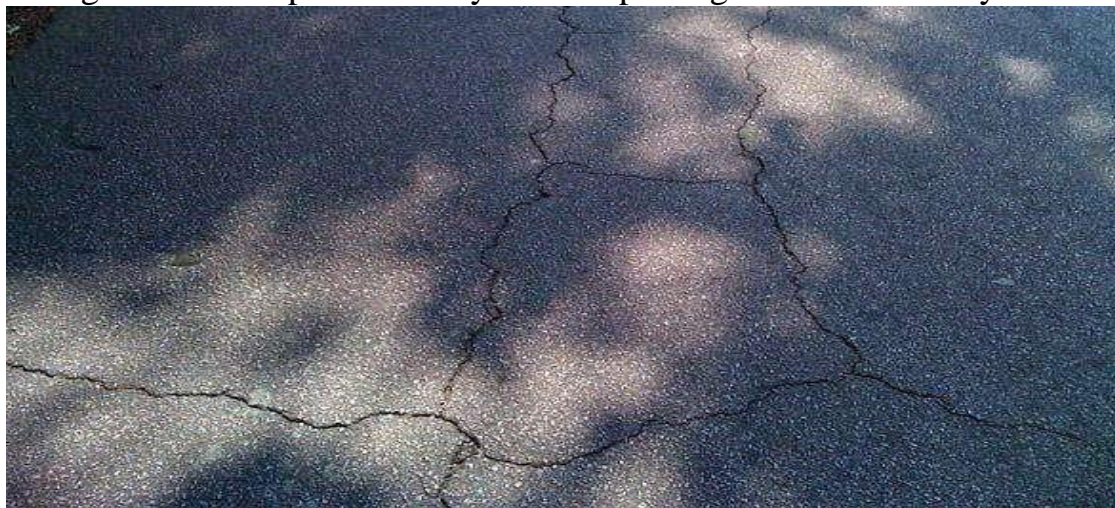
Fig. Block Cracking
